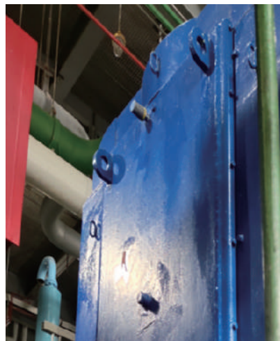
Condensate Pump Monitoring – Power Plant
