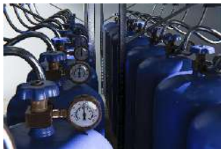
Alarm for Hydro Pneumatic Tank
